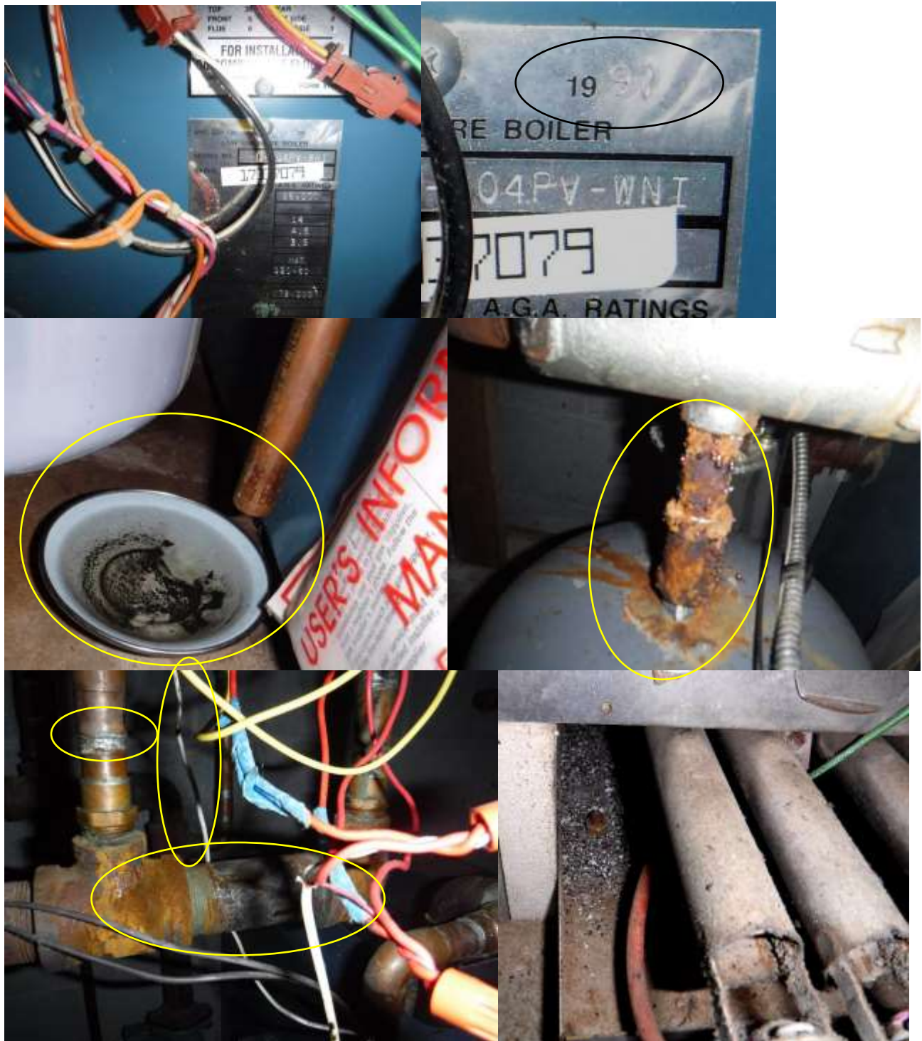
Figure 34 Scorch marks on plastic wire sheathing near patched copper piping/solder. Piping on boiler had corrosion and dissimilar metals (galvanized and copper) and no dielectric insulators/unions; improper. Boiler was leaking, corrosion, soot & rust particulates on burners, etc.; past life and poor condition. Home was not properly winterized and water visible in ruptured baseboards throughout the home.
