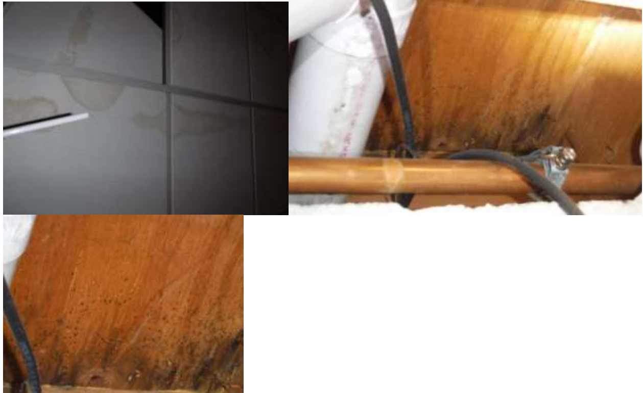
Figure 30 Leaks and mold like substances in basement or in the home. Further evaluate by a mold contractor. See heating & plumbing section comments.
