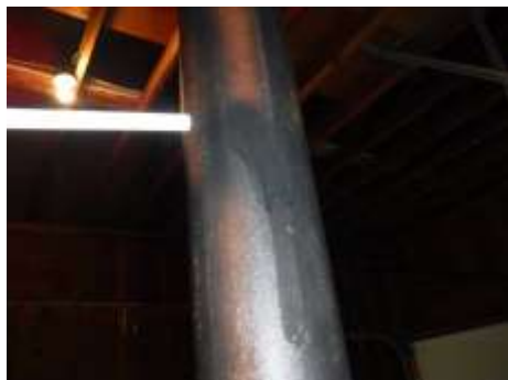
Figure 11 The lally column was covered in condensation/weeping; have evaluated. Condensation or wicking inside lally columns can deteriorate these structural supports.
