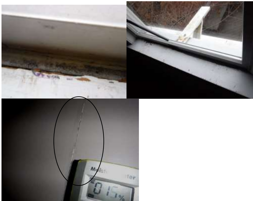
Figure 21 Leaking around the windows, cracks on drywall and active moisture. All black staining or mold like areas in the home should be evaluated by a mold or environmental contractor.
