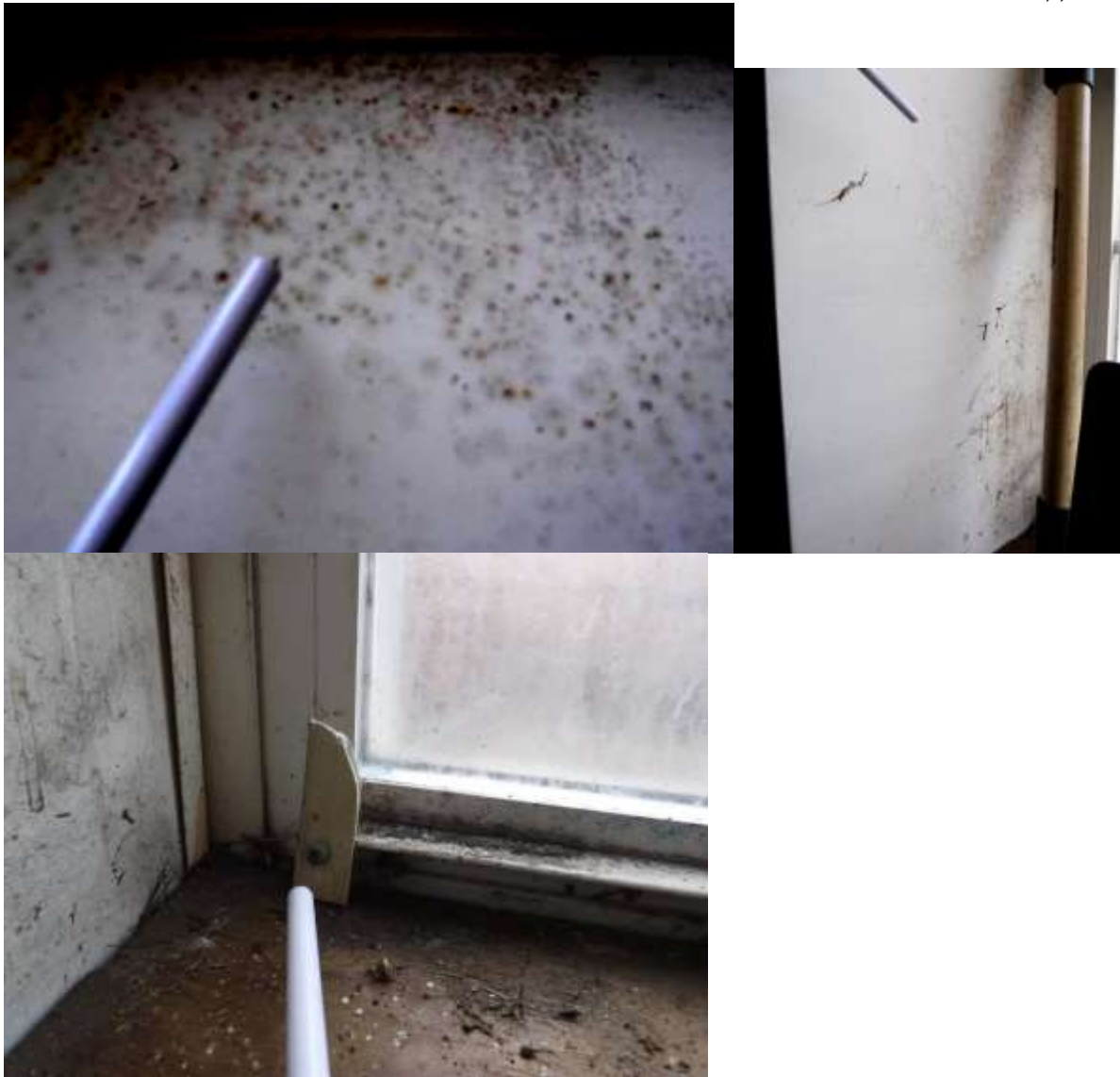
Figure 28 Mold-like spotting/staining; follow up with a mold/environmental contractor for mold evaluation ( beyond scope of a home inspection).
