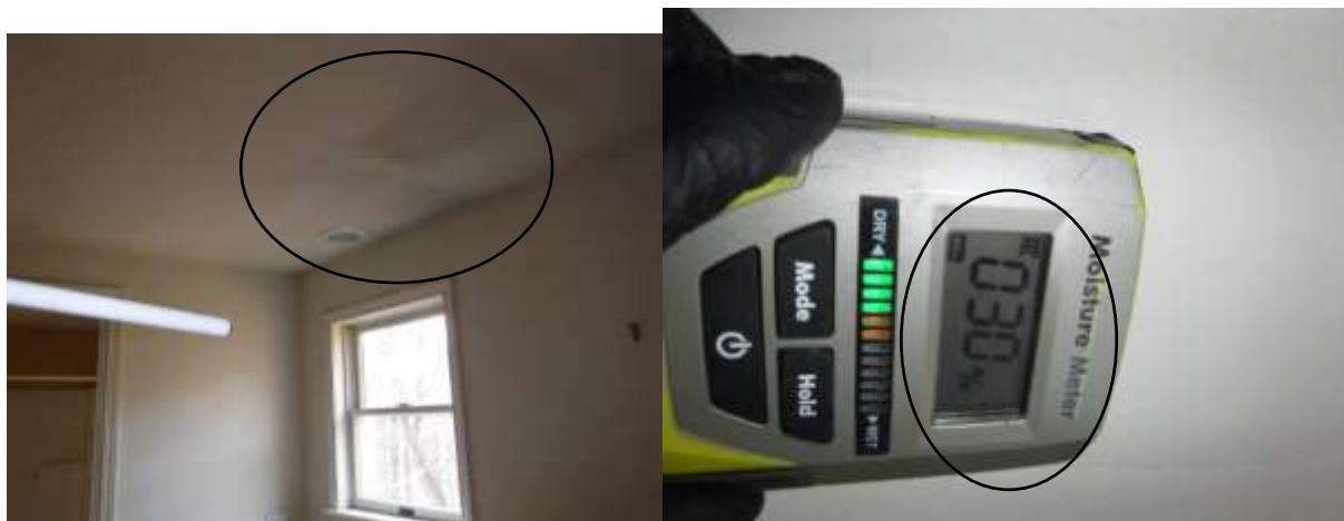
Figure 18 Active leaking in the home; roof, plumbing and heating water sources. The home was poorly maintained and not properly winterized.
