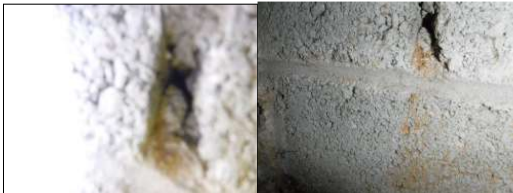
Figure 27 Termite tubes inside a gap in the foundation wall in basement. See separate NPMA-33 termite report.
