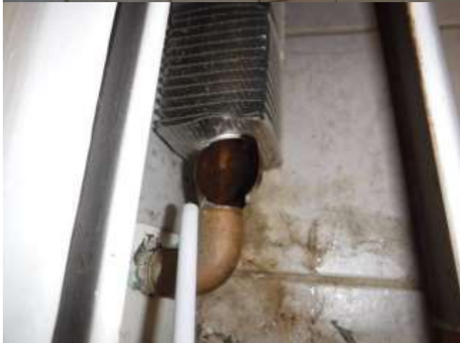
Figure 19 View of ruptured baseboard in bathroom. There were many throughout the home. The home was not winterized properly. See heating & plumbing section comments.
