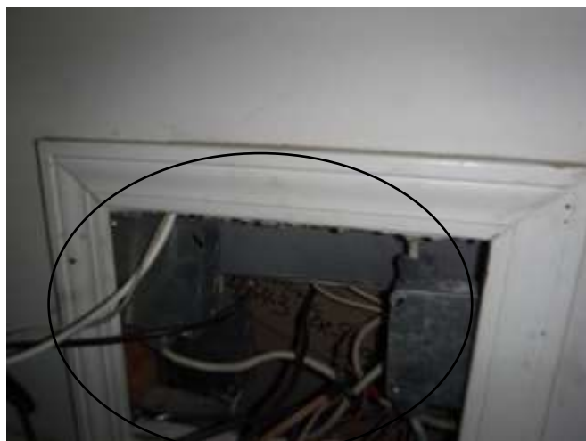
Figure 24 Electrical wiring inside wall; safety concerns. Recommend an electrician evaluate & repair.
