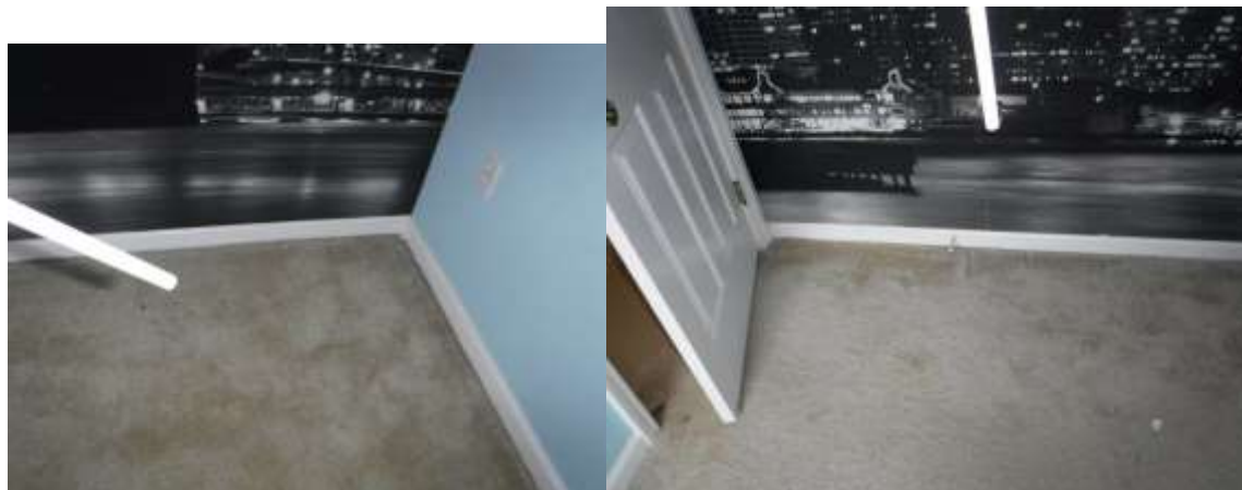
Figure 25 Sloped flooring, squeaking, and deflection or bounce when walked upon flooring.
