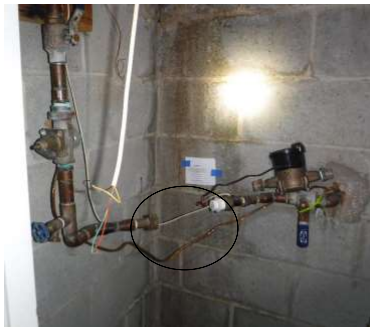
Figure 33 Water meter was apart and plugged on street side.
