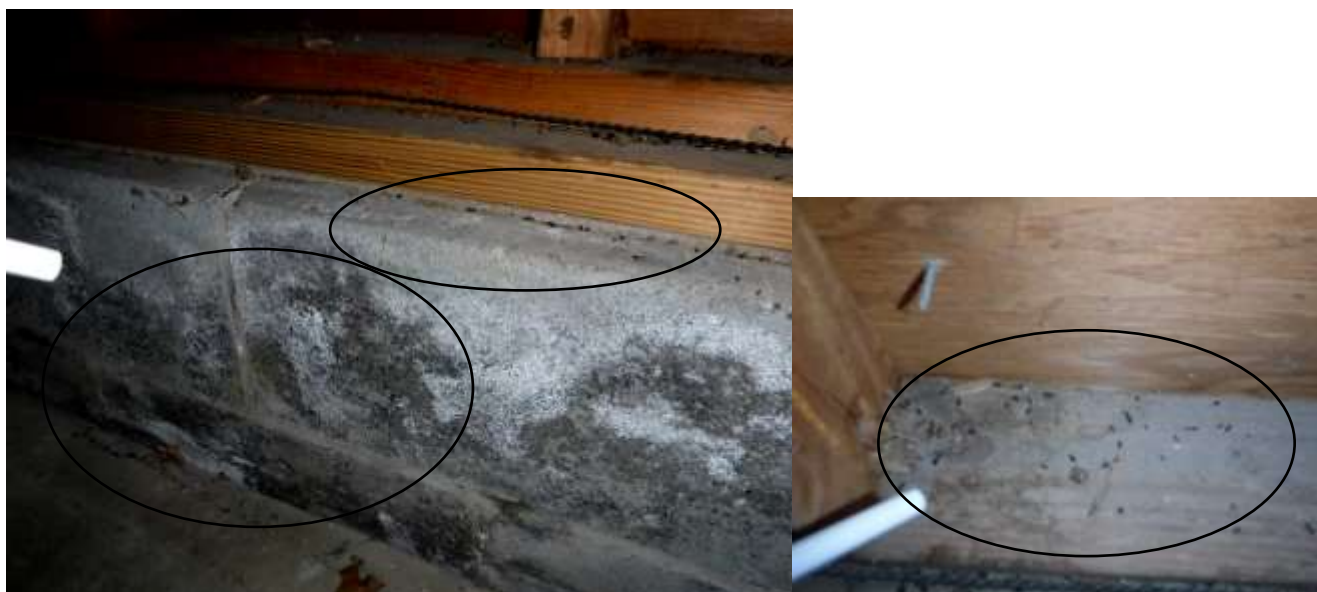
Figure 12 Example of efflorescence, water stains, seepage. The driveway drains toward the garage and grading & drainage needs to be corrected; negative grading. There were mice droppings in garage and in the home; have all gaps, daylight, openings and crevices sealed to maintain seals for water, insects and rodents.
