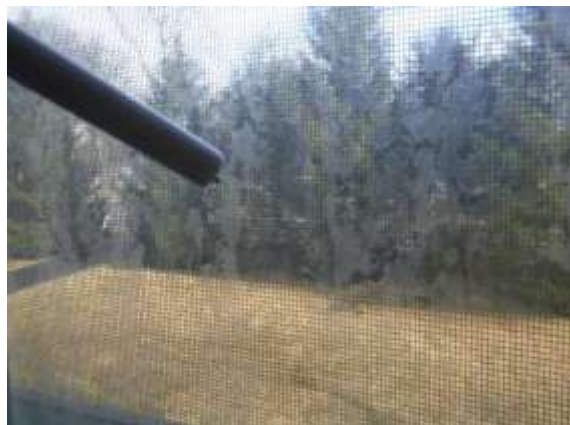
Figure 16 Example of vapor seal breaks have window in home evaluated for replacement.
