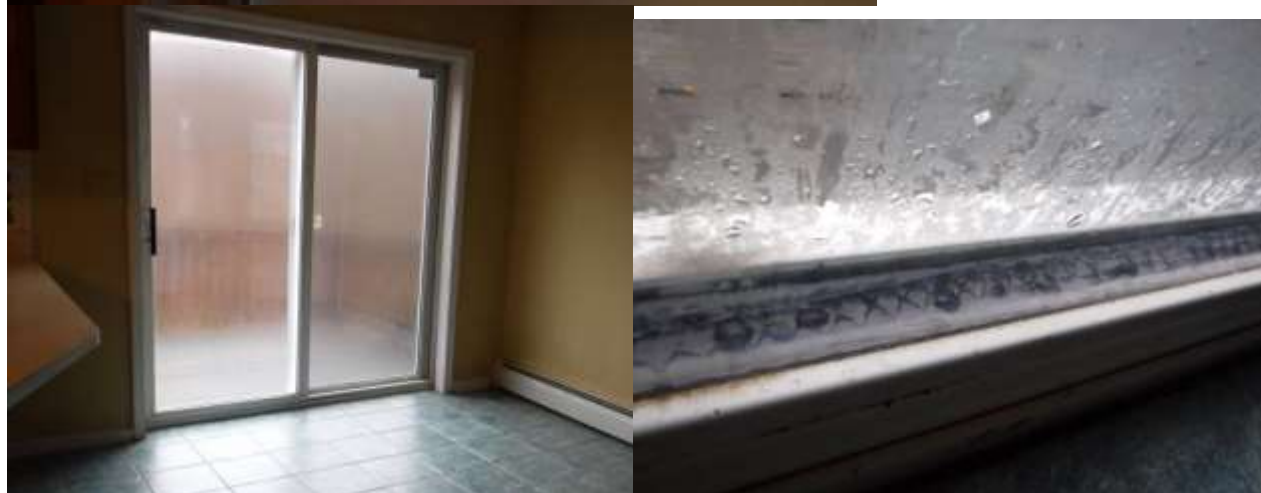
Figure 15 Windows and doors throughout the home were in poor condition. There was broken glass on window(s) and vapor seal breaks; have replaced throughout the home.
