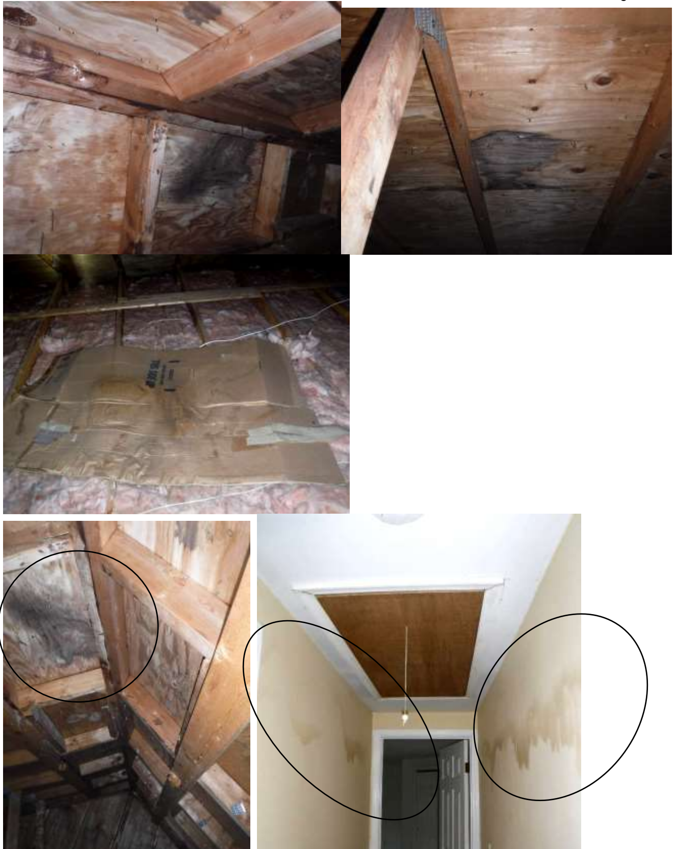
Figure 8 Examples of water stains/leaks in attic. See other sections comments; active leaks in home.
