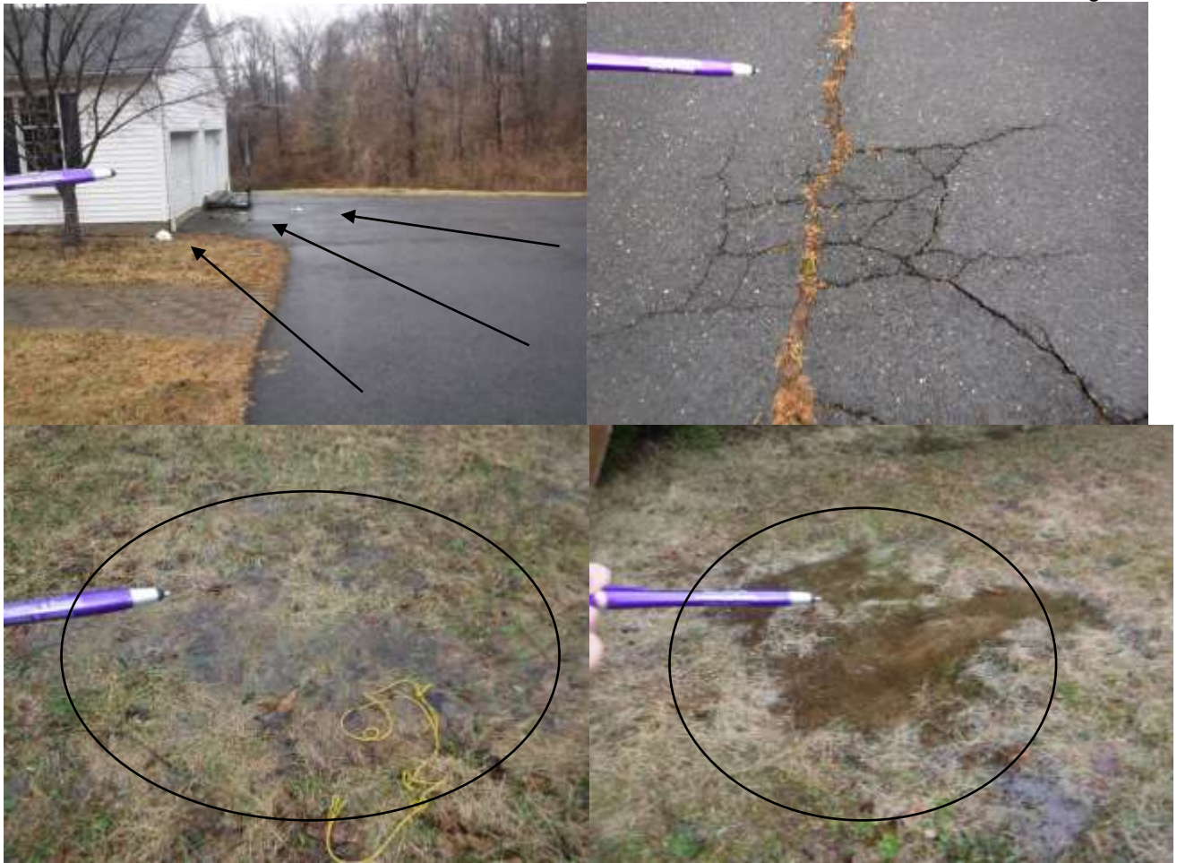
Figure 4 Example of drainage concerns. Water drains off the driveway towards the garage and ponding in the yard. The driveway had water damage, deep cracks and no drainage across the garage.
