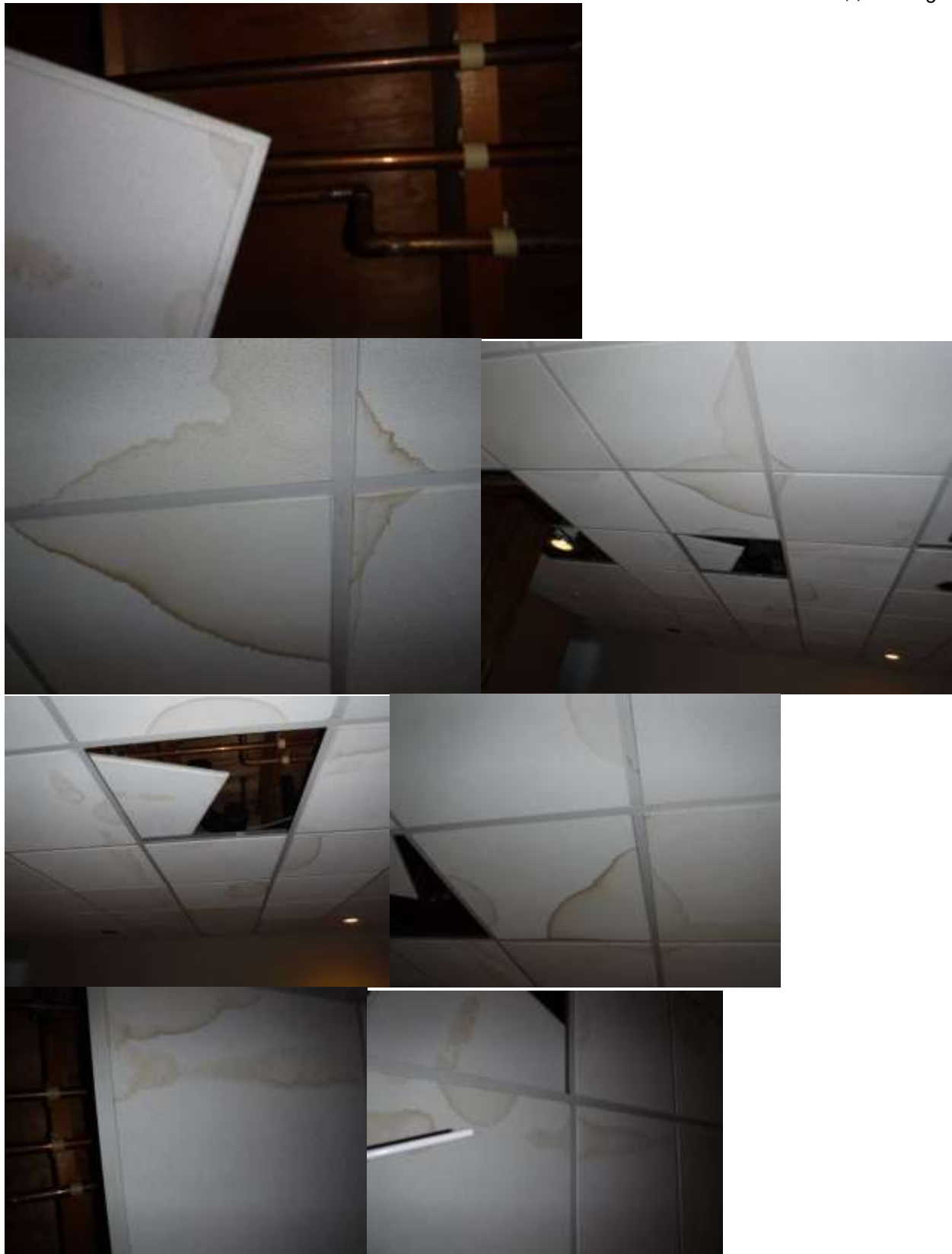
Figure 29 Examples of ceilings that were found partially opened in the basement, water stains/leaks and plumbing exposed. The home was not properly winterized and leaking active throughout the home.
