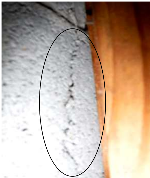
Figure 31 Example of foundation cracks. Limited view due to finished basement. Recommend a structural engineer (PE) and building contractor further evaluate all foundation cracks and advise on repairs before closing.
