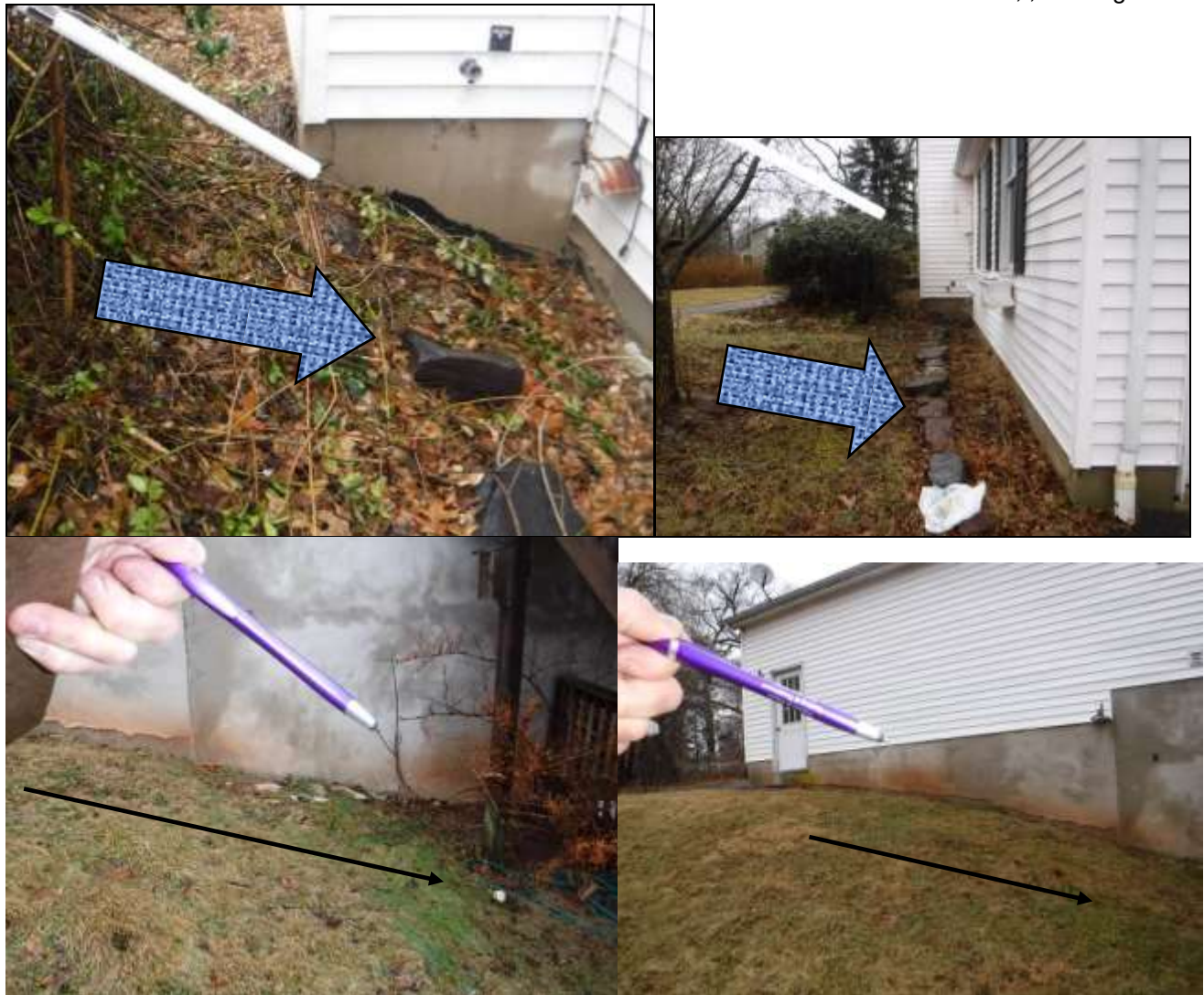
Figure 2 Examples of negative grading and erosion; water drains toward the foundation/basement. There was observed seepage in the basement and garage. Recommend a grading & drainage contractor and wet basement contractor evaluate and advise on grading & drainage and water management systems.
