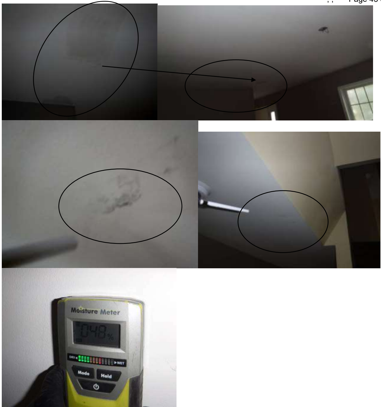
Figure 23 Active leaking in ceiling by living room and front entrance. There were ruptured baseboards above on second floor with water inside them.
