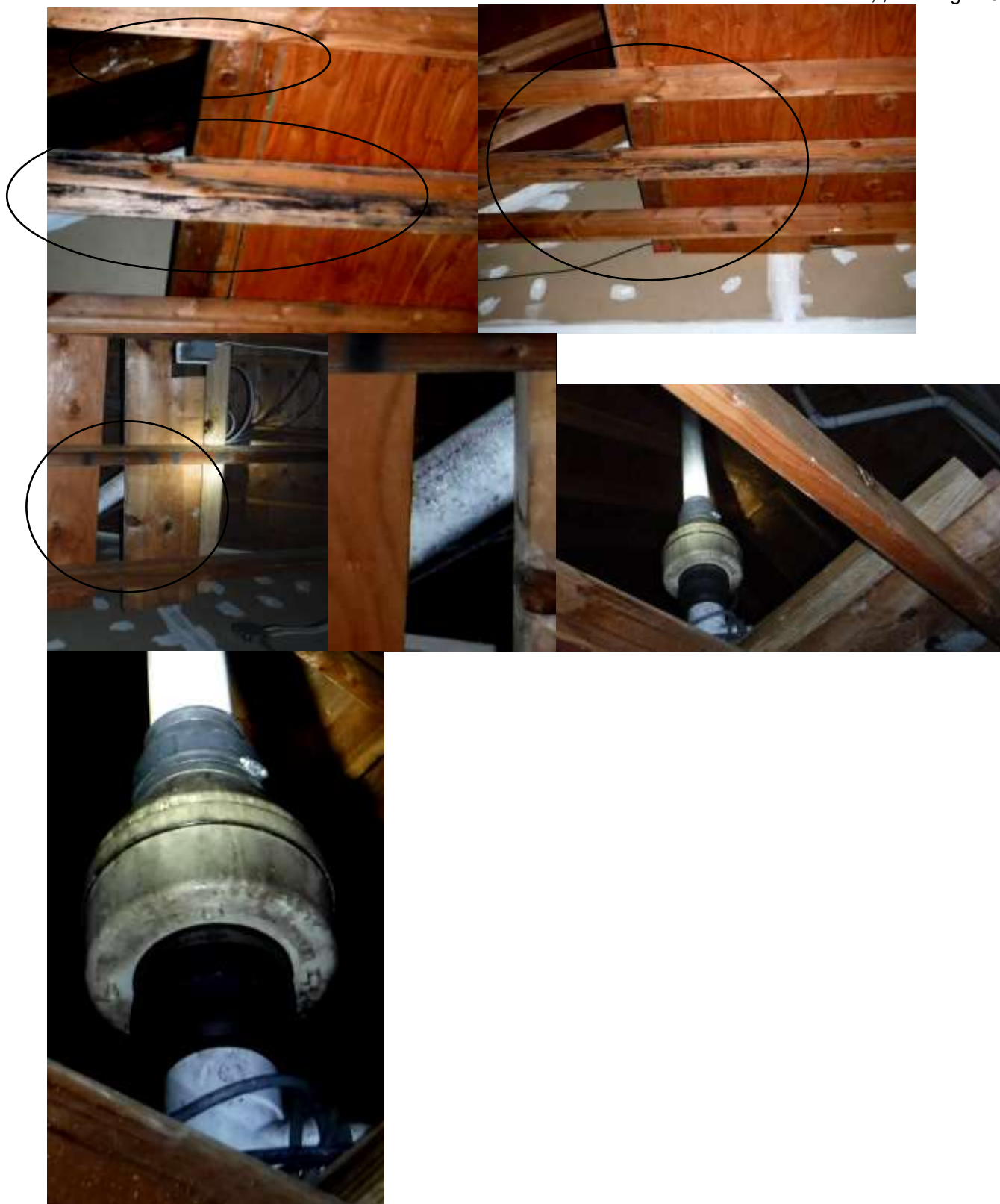
Figure 10 Example of dark/black staining on rafters or roof lumber and radon system and water stains around the radon system on 2x4s; mold like. Recommend a mold/environmental contractor evaluate and advise on mold testing.
