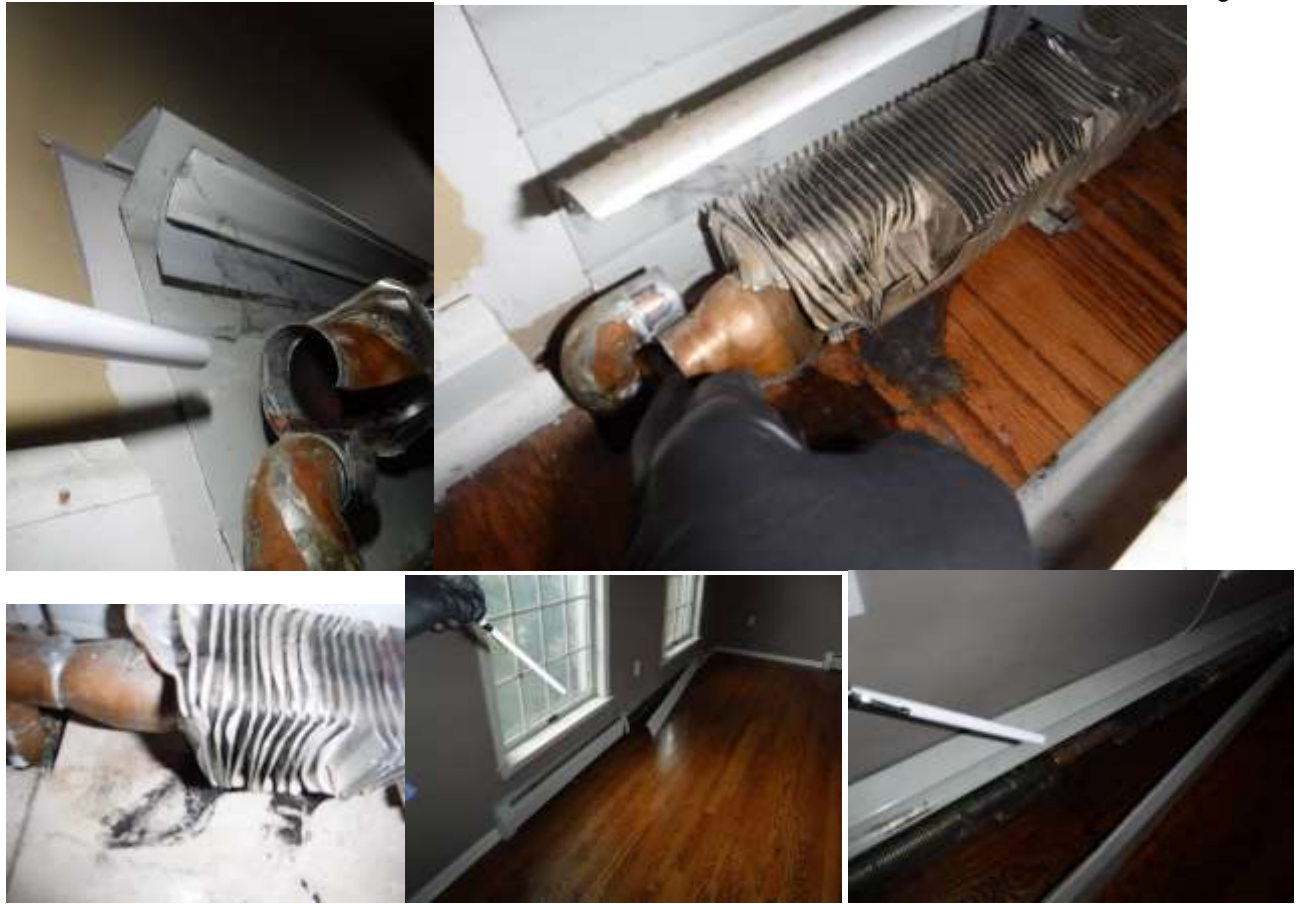
Figure 22 Example of many baseboard that had ruptured due to freeze damage; active leaking. See heating section comments.
