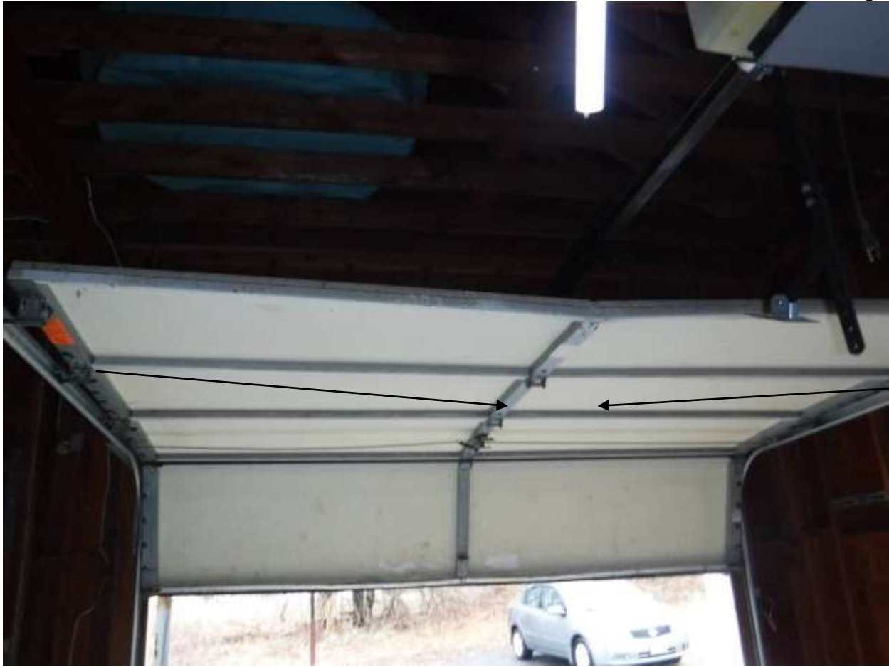
Figure 14 Damaged door panels; have evaluated for replacements. The doors were misaligned, not locking, daylight around doors, damaged locks, door openers unplugged/not working, not plumb, etc.
