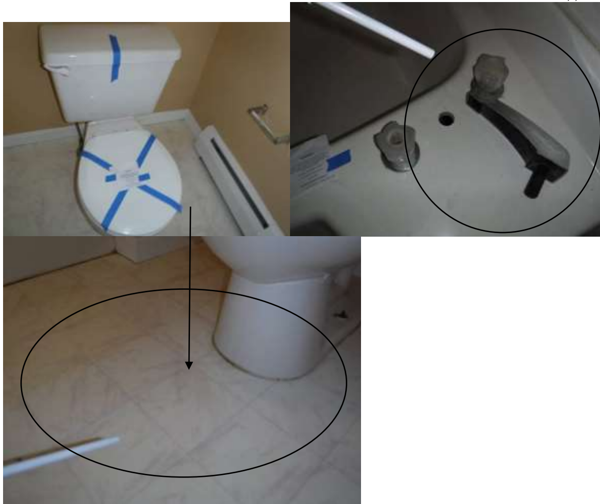
Figure 17 Water puddle on floor around the toilet; leaking plumbing and heating baseboards in the home; freeze damage/improperly winterized and the meter was found removed and plugged on street side in basement.
