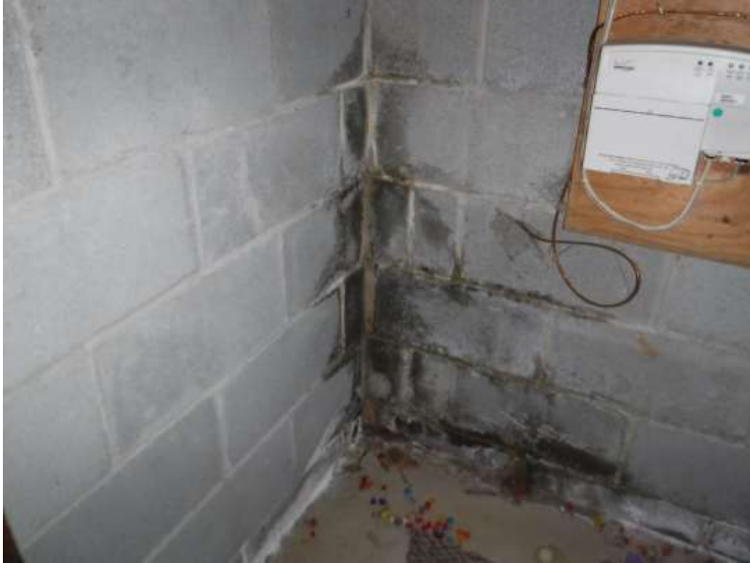
Figure 32 Example of seepage in basement; limited access by mechanicals or utility areas.
