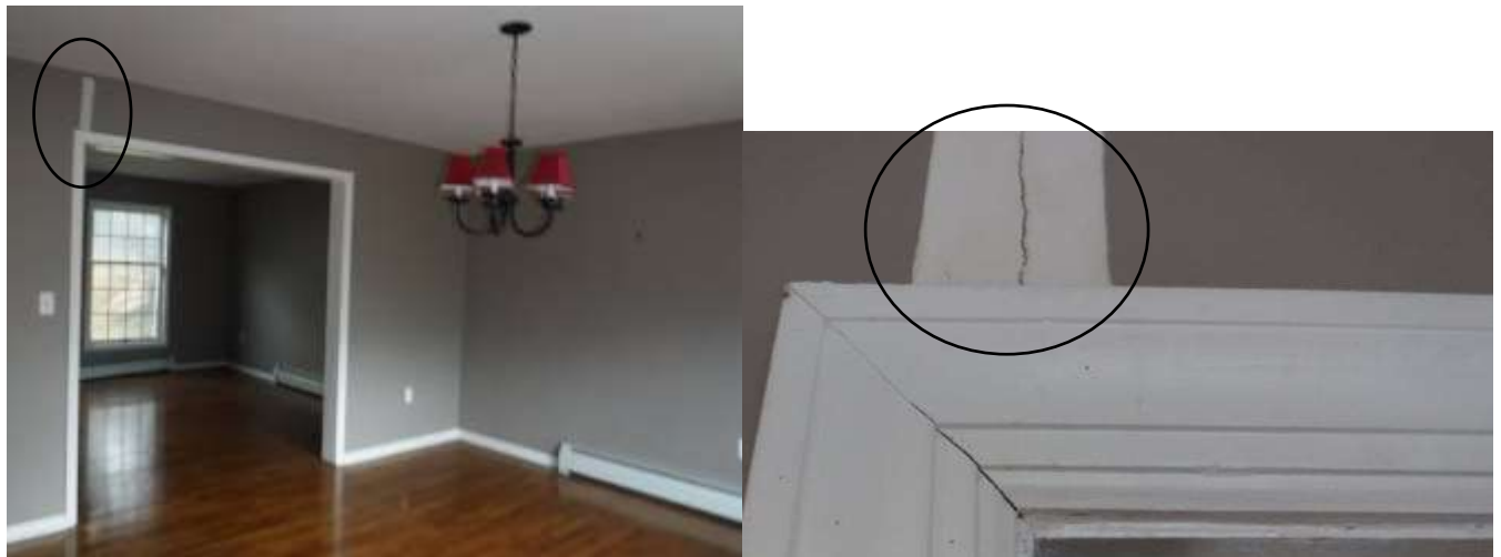
Figure 20 Have a building contractor evaluate the canted doorway and vertical cracks.
