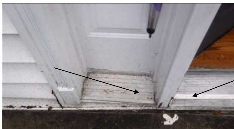
Figure 3 The front door assembly was damaged; have a building contractor evaluate for replacement including concealed damage.
