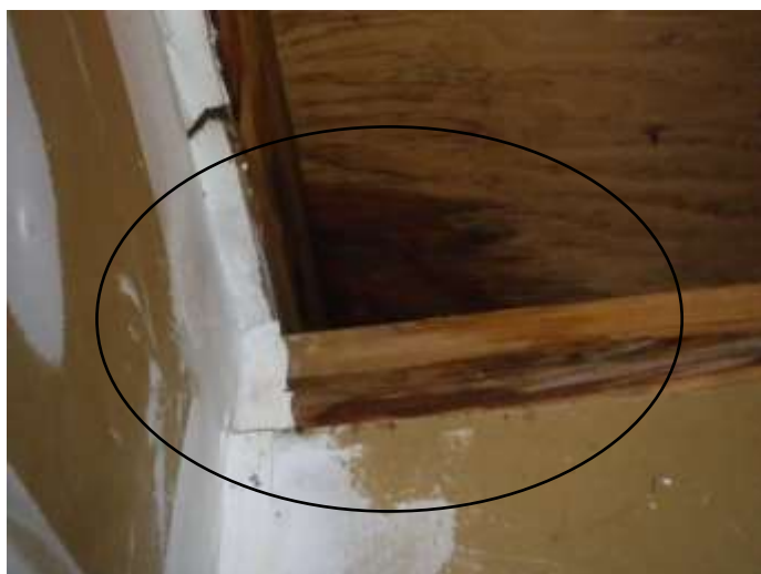
Figure 13 Example of active roof leaks; see roofing section comments.
